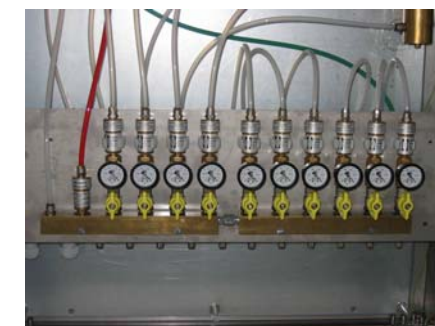
Manifold outlets for each pipe section to be monitored
