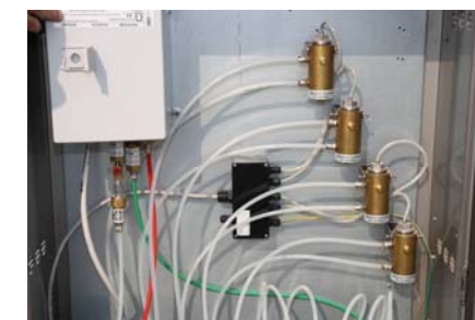
Sensors for pressure pipe leak detection
